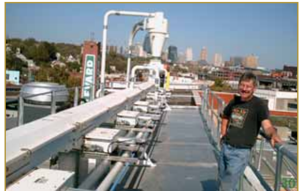
Installation of roof top mounted 9SWRs. Conveyors move whole malt grains and is equipped with 7 intermediate air-operated discharge gates with chain wipers.
